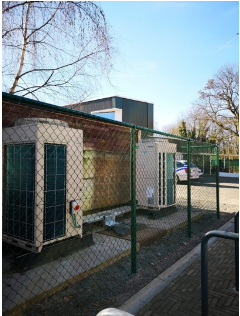
HVAC and SANITARY Office building Heating and cooling with VRV Collective air groups Building work
